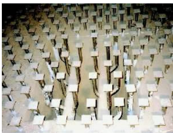
Improved bottom ash removal as a result of BFB boiler conversion
