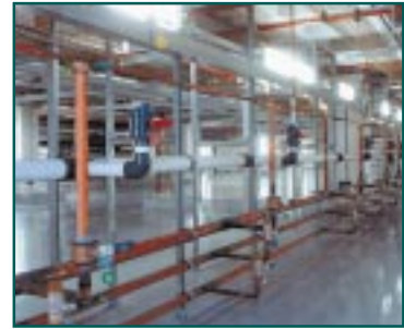
Utility services for cleanroom.
