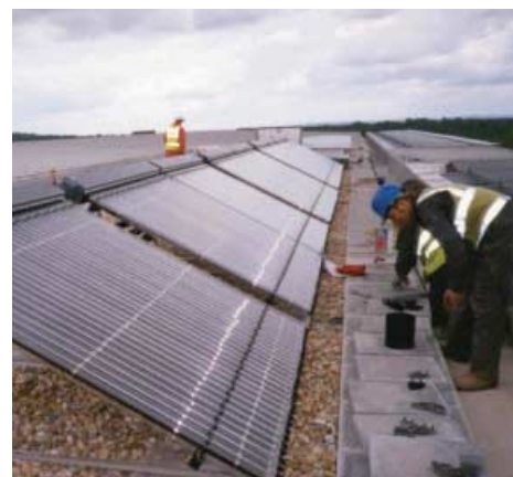
30 m 2 of solar evacuated tube collectors for a new office development in Belfast
