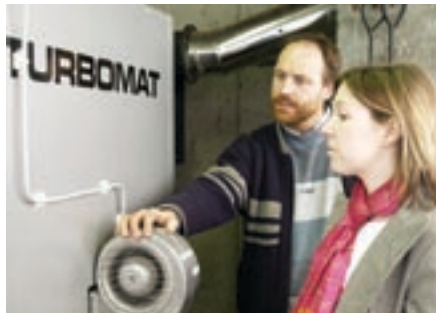
Left to right, pictured in the wood chip boiler house at Camphill's Jerpoint Centre, John O'Connor, Manager Camphill and Aine Carr, SEI
