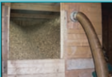
Wood chips are blown into fuel bunker.
