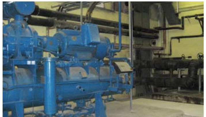
One of the screw compressors operating on the Chilled Water System at Kerry Ingredients Charleville.
