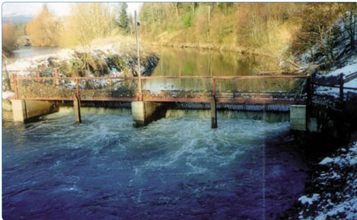
Fixed screen installation at point of return of tailrace flow to main river. This screen will prevent the entry of upstream migrating salmon entering the tailrace.
