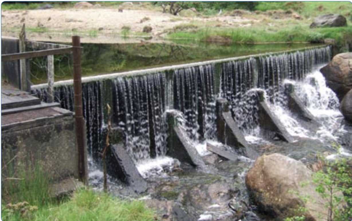
Obstruction to upstream fish passage.
