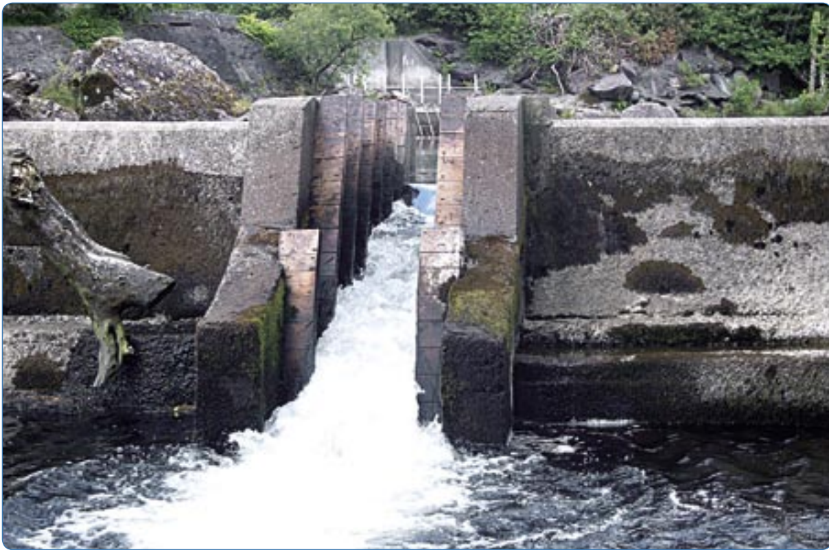
Denil fish pass to allow upstream movement of fish.
