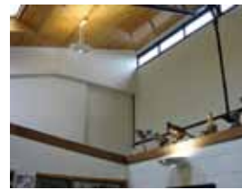
Fig.7 Poor luminaire positioning wastes energy
