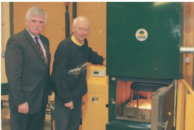
James Kennedy, NPS and Bernard Rice, Teagasc, pictured with the wood chip boiler installed at Teagasc.
