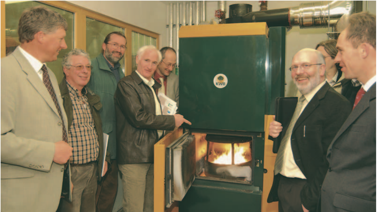
SEI Site Visit to the Coillte Wood Pellet Boiler, Newtownmountkennedy, Co. Wicklow
